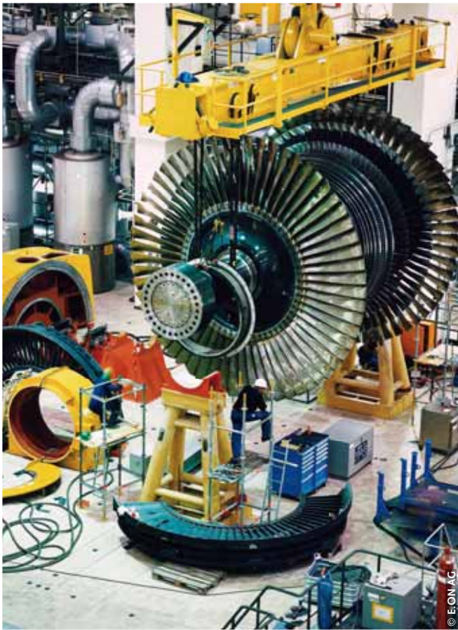
Turbine in nuclear power plant
