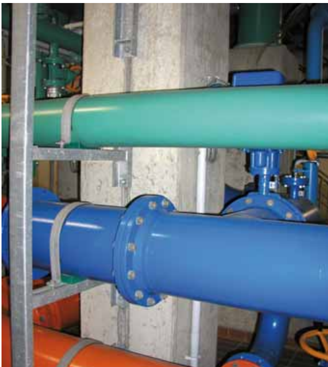
Pipe support using vertical channel
