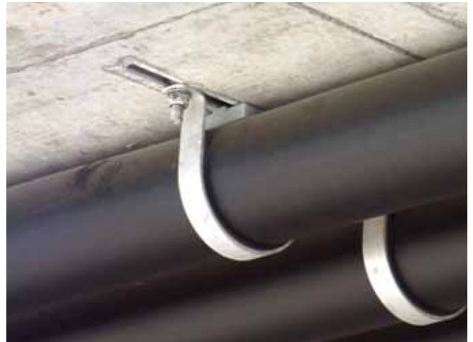
Pipe support bolted to ceiling
